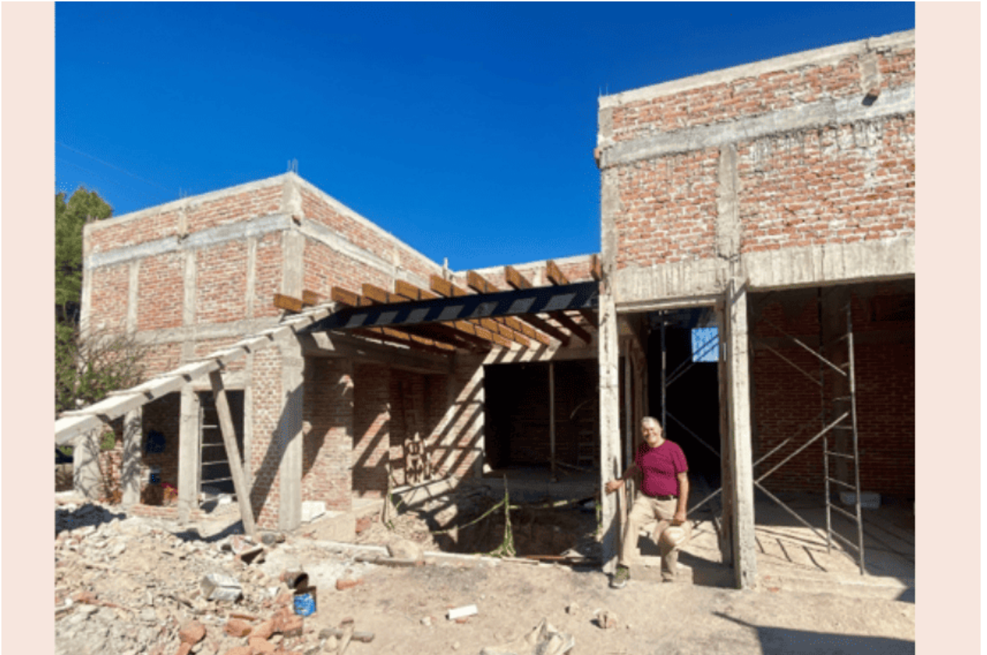
Lee Carter, co-founder of Mitigare Cuidados Paliativos A.C., at the construction site in San Miguel de Allende.
